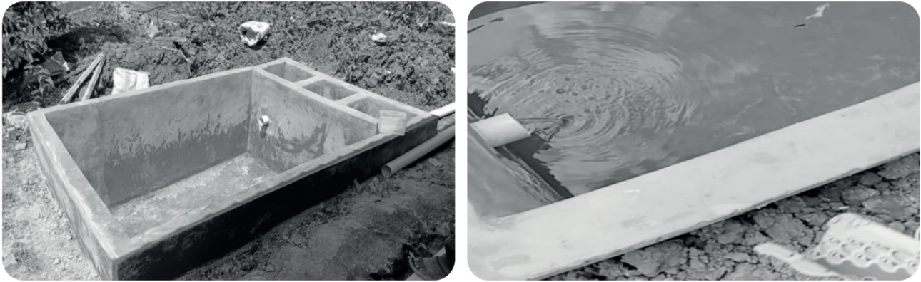
Figure 4: Water filtration pool. Source: Irmawanty and Syam, 2024.
